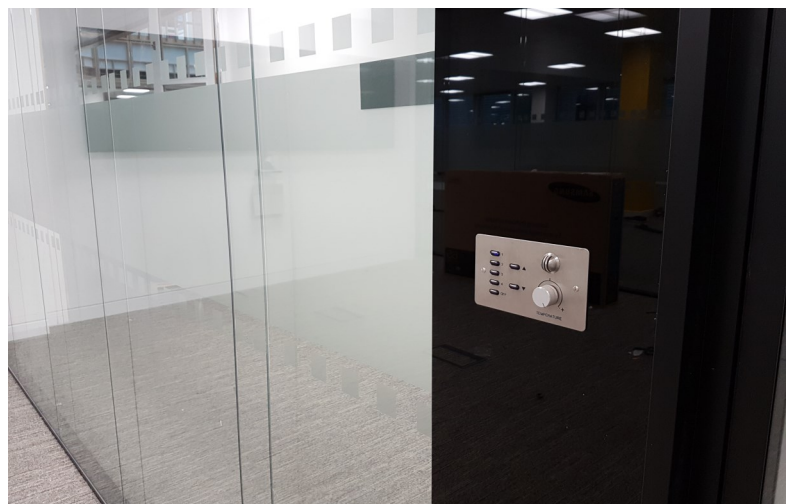
Custom Scene Plate installed on one of our sites, Wimbledon Bridge House (above).
